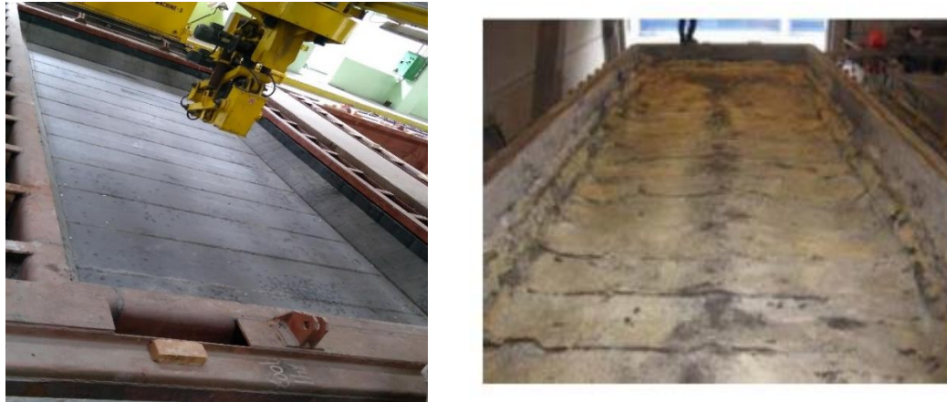
Figure 2. Left: newly lined pot lining, Right: dead pot lining.
